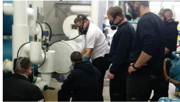
Town of Caledon Respirator Fit Testing and Arena Plant Room Training Photo – Note: Different masks are being used as part of the educational process
